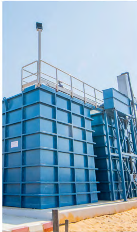
Sewage Treatment Units
