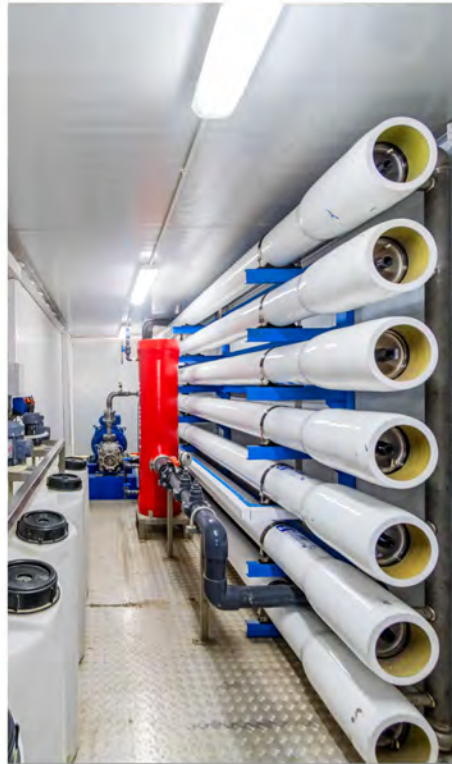
Containerized Reverse Osmosis
