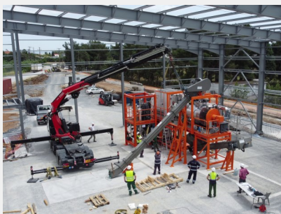
Installation of mobile VacuDry® plant
